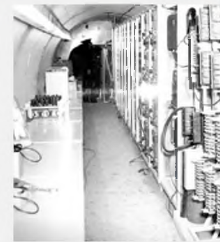
Data interception equipment stationed in the tunnel
